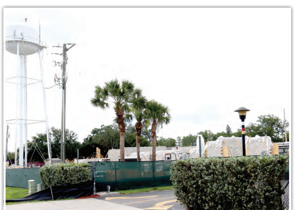
Kevin Johnson NEW DIGS: The academic year has ended at Ahfachkee, but the construction work continues for the school's expansion project.
