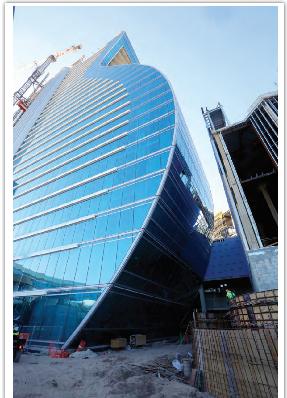
VIEW FROM ABOVE AND BELOW: Above, here's the view March 6 from near the top of the new guitar-shaped hotel being built at the Seminole Hard Rock Hotel & Casino Hollywood. At right, a look up at the hotel from ground level. The hotel is scheduled to open this fall. According to a Hard Rock press release, the expansion will include "638 luxury guestrooms to a first-ever, iconic, guitar-shaped hotel and 168 upscale guest accommodations in an adjacent hotel tower overlooking a lush, "Bora Bora" style, private cabana environment..."
