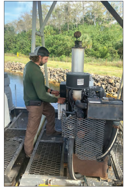
Courtesy photo Chris Self, ERMD water master, runs the E2 pump in Big Cypress in October.
