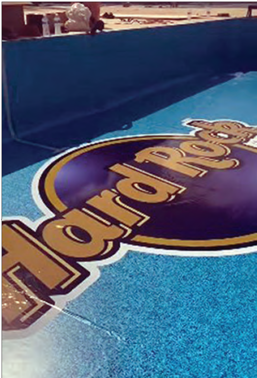
COOL POOL: Finishing touches are made to a swimming pool that is part of the Hard Rock Beach Club at the Miami International Autodrome racetrack on the Hard Rock Stadium campus in Miami Gardens. The track will host the Miami Grand Prix Formula 1 race May 8. The club is set up near one of the turns on the track. Its features include pools, sand and cabanas.
