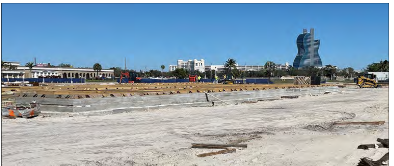
CONSTRUCTION SCENES: Several big construction projects are underway on the tribe's reservations, including the Seminole Casino Hotel Brighton on the Brighton Reservation (above on Feb. 16) and a new preschool on the Hollywood Reservation (below on Feb. 20).
